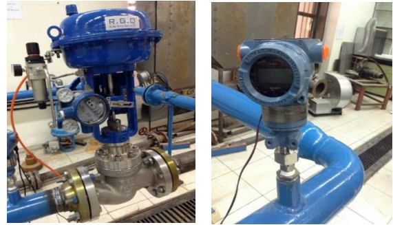
Figure 5- Valve installed in 3-in pipeline (left), Pressure transducers installed on pressure taps (right)
