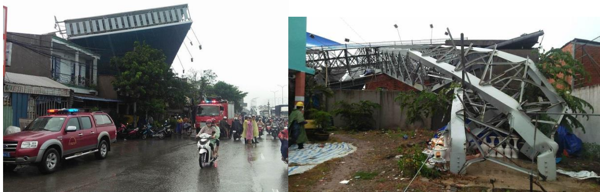
Figure 1. Damage of Billboard and partial damage building (Highway 1A, Binh Tan district, Ho Chi Minh city, 10 August 2018) [2]
