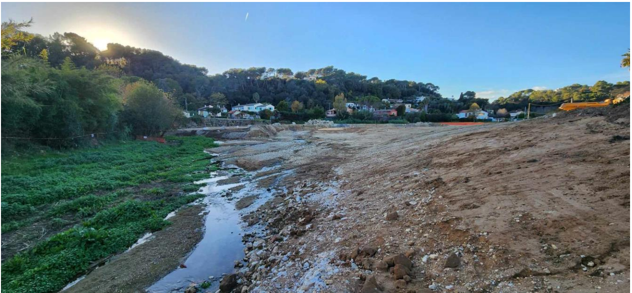
Figure 2: Photo of restructuring of the Brague main channel taken on 11/29/2023 near the hydrometric station at Biot.
