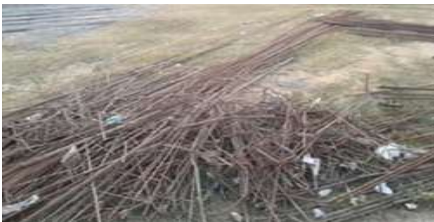
Fig. 4. Steel Waste on Site (Current State)
